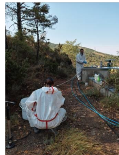
B2.1 Barrier area – soda injection
